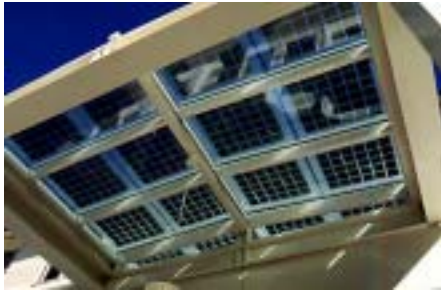
Fig 4: Laminated Photovoltaic glazing at the Thoreau Center generates electricity while filtering daylight through this entry.
